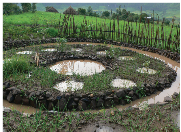
Figure 5: Ring basin infiltration pit, Dehana Woreda, Gaqiew village. Photo: HELVETAS / Firiehiwot Yibeltal-2016
